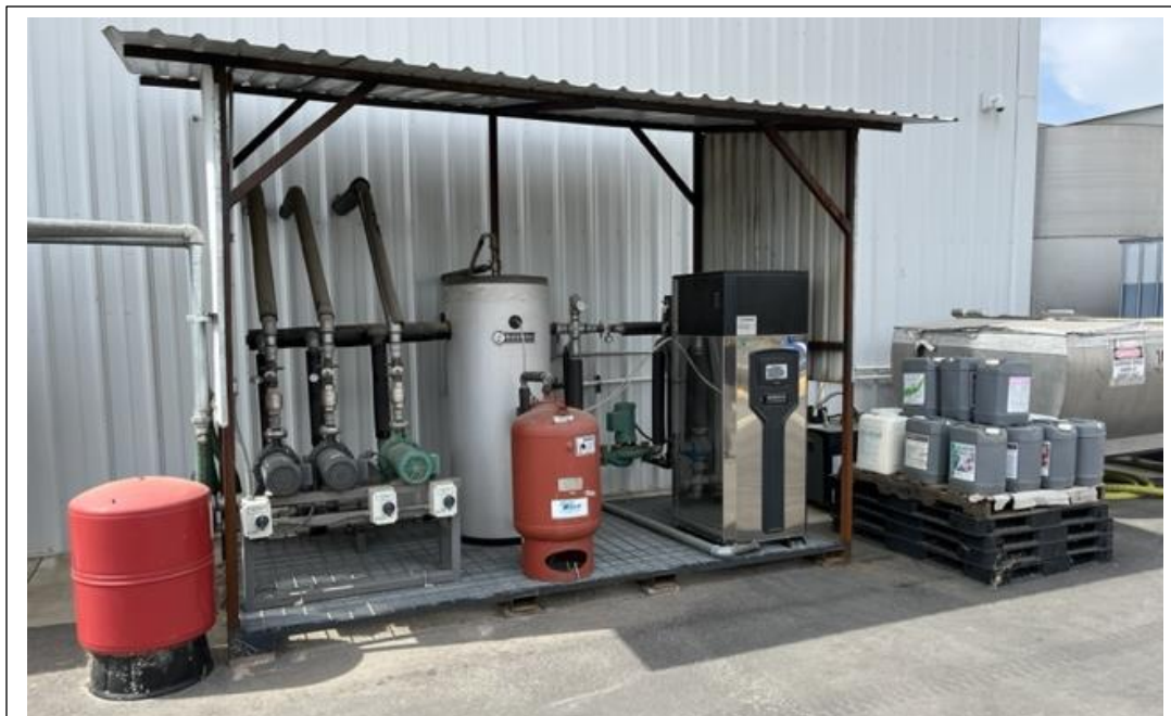
Water heater for generating hot water piped to indoor mixing tanks.
