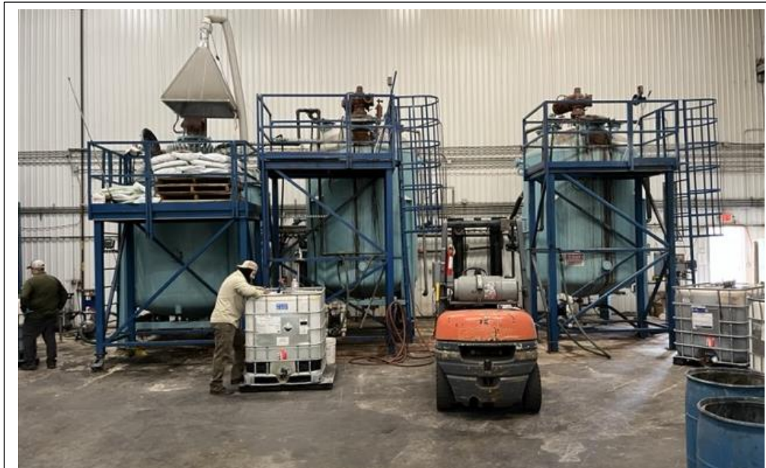
Baghouse operation inside manufacturing facility. Dust and particles are captured with not outside release.
