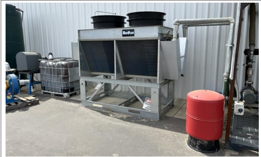
Outside filter system connected to indoor baghouse.
