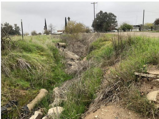
Figure 5 On southwest corner of Travers Creek, facing west towards the roadside ditch
