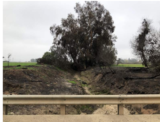
Figure 4 On existing bridge, looking downstream. Please note, parts of the creek damaged by a fire.
