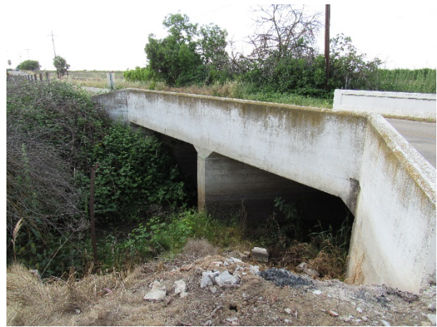
Travers Creek / E Parlier Avenue Caltrans Bridge No: 42C0684 Fresno County Bridge No: 10-099
