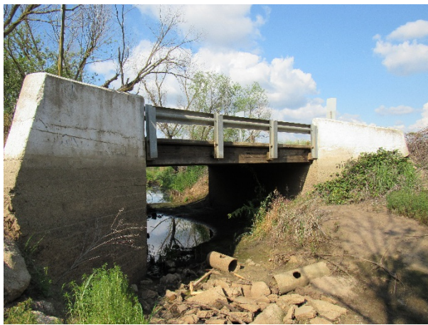
Travers Creek / E Lincoln Avenue Caltrans Bridge No: 420683 Fresno County Bridge No: 10-065
