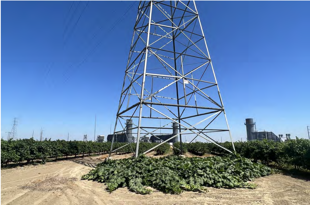
Photograph 5. Schindler-Panoche 115 kV Transmission Line, View North.
