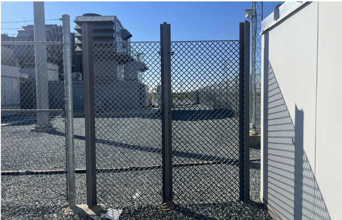
Figure 8 Midway Peaker Plant Within Study Area, View South
