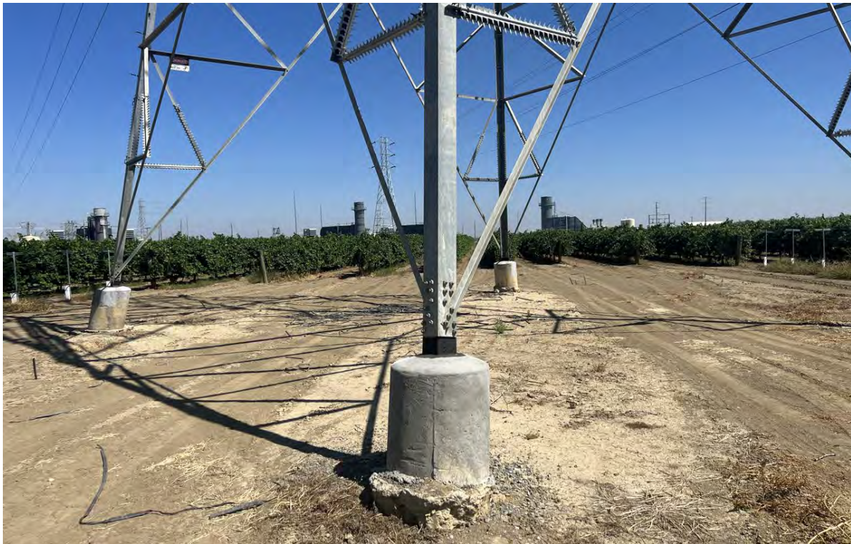
Photograph 6. Panoche Kearney 230 kV Transmission Line, View North.
