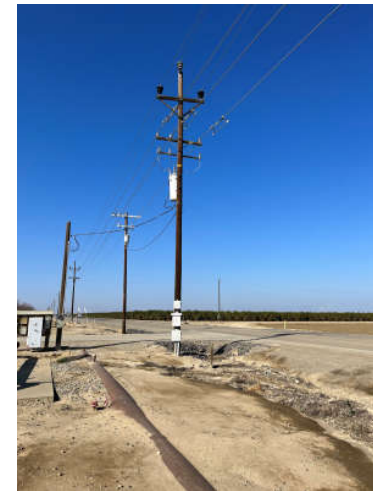
Photograph 4. View of a pole-mounted transformer on the northwestern corner of the subject property.
