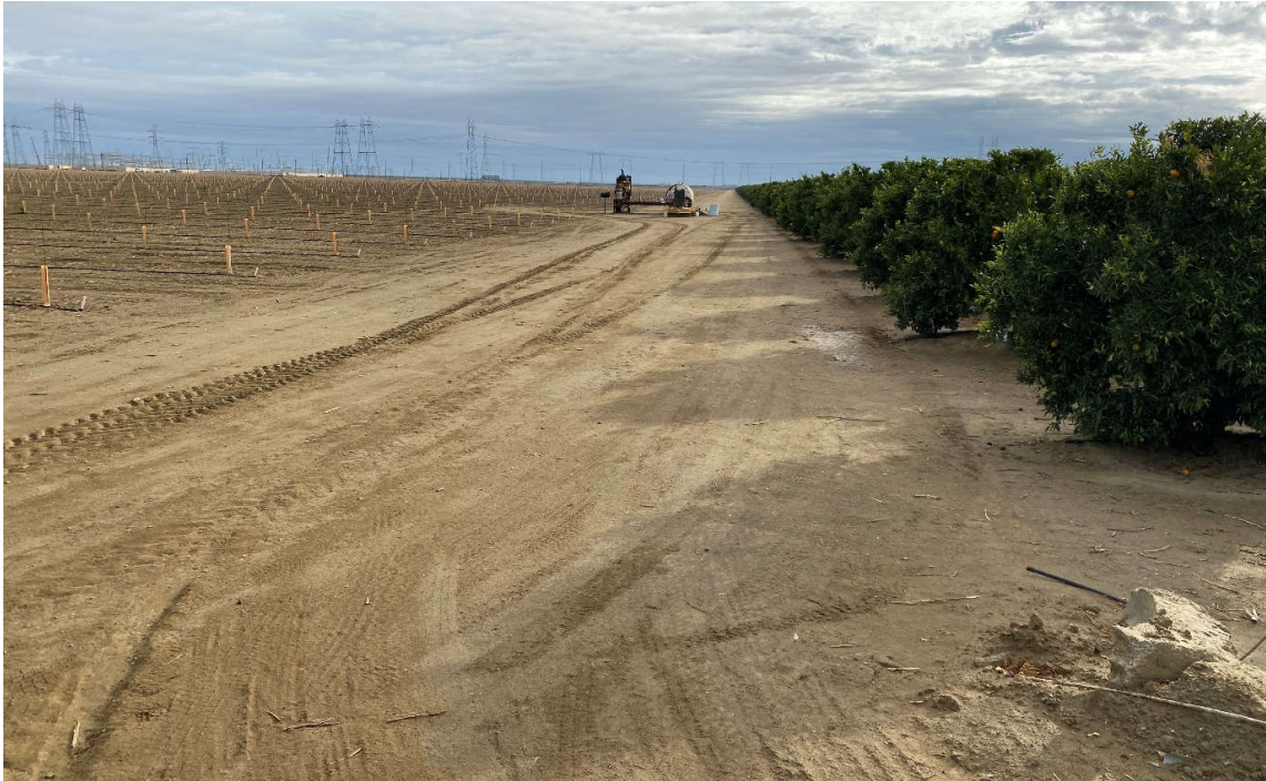
Photograph 3. Compacted dirt road with active agriculture on left and orchard grove on right. View east. November 9, 2021.
