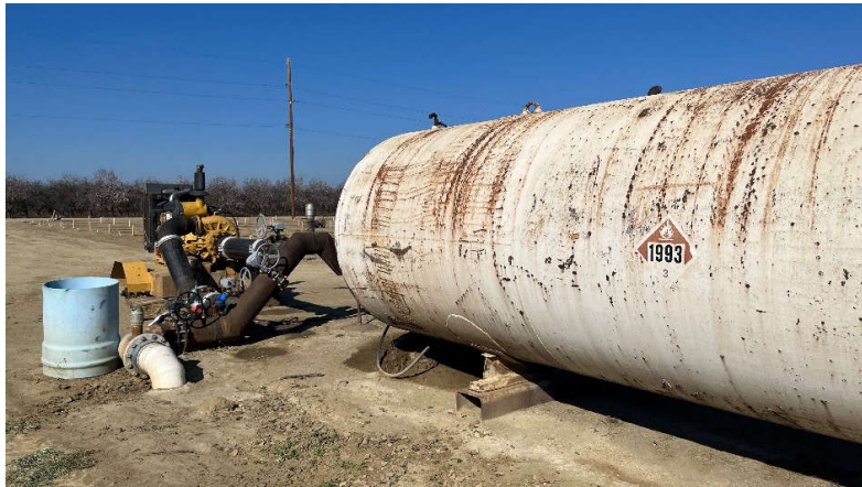
Photograph 5. View of the diesel AST and associated machinery observed on the western portion of Parcel 085-040-58S.
