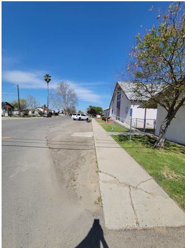
Figure 10: NE side of Quince facing NW from the NW elementary school entrance.
